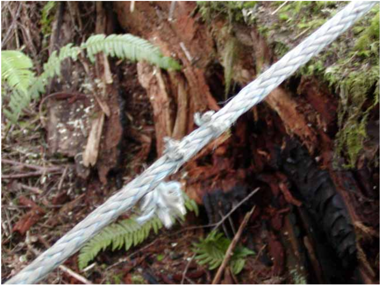
Figure R10. Tail tree guyline with partial cuts in a couple of non-adjacent strands. While this situation does not exceed manufacturer's out of service criteria, removal and re-splicing (long splice) of this section would be a prudent action by the operator.
